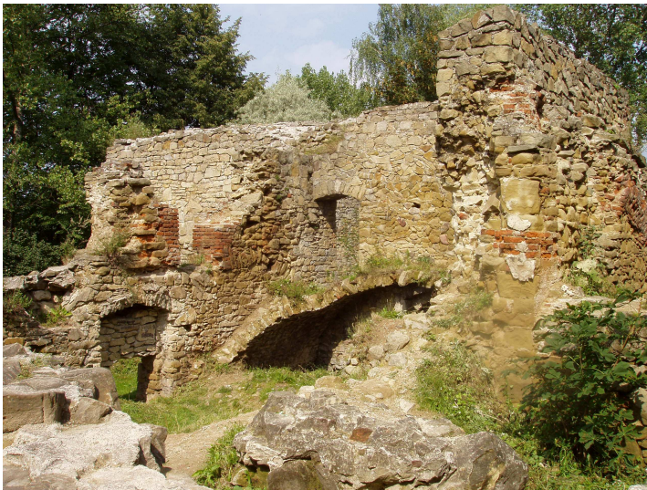
Part of the ruins of a medieval castle, on the bank of the river Dunajec
